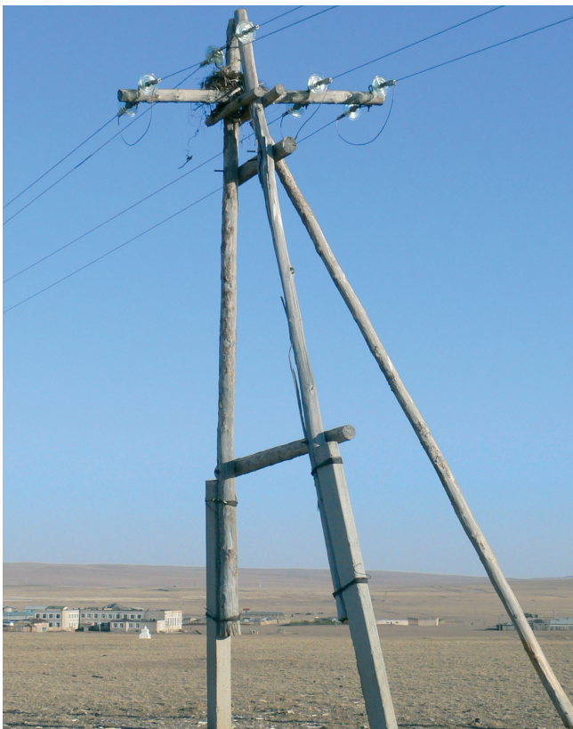
Figure 2. Nest of Raven built in a dangerous position on an electricity distribution line. Note trailing wires from nest structure.
