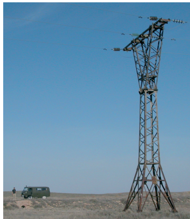
Figure 5. Survey of power lines in the Betpaqdala desert (A. Levin).
