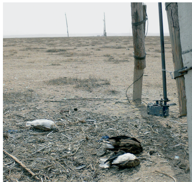
Figure 3. Three Upland Buzzards electrocuted at poorly designed junction point along a distribution line.
