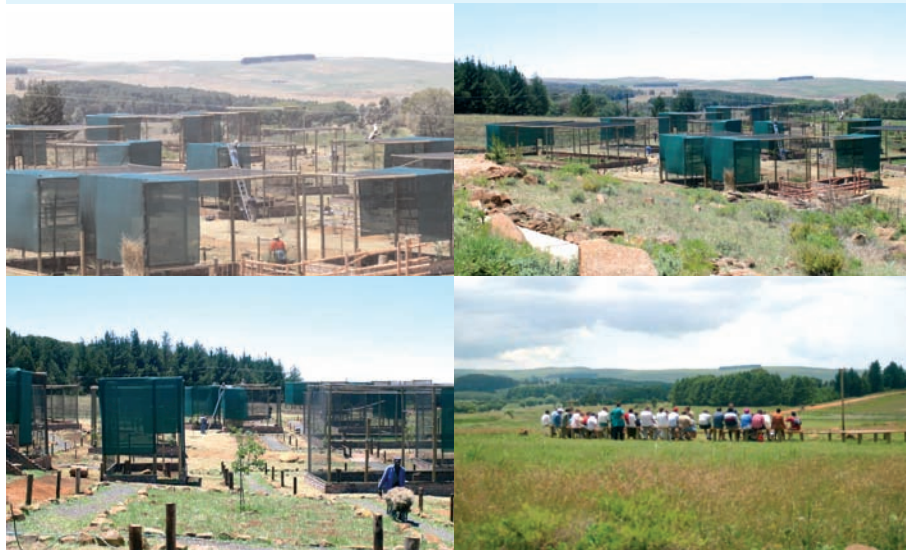
■ clockwise, from left: work underway, constructing the aviaries, building with help from the locals, demonstration in progress
