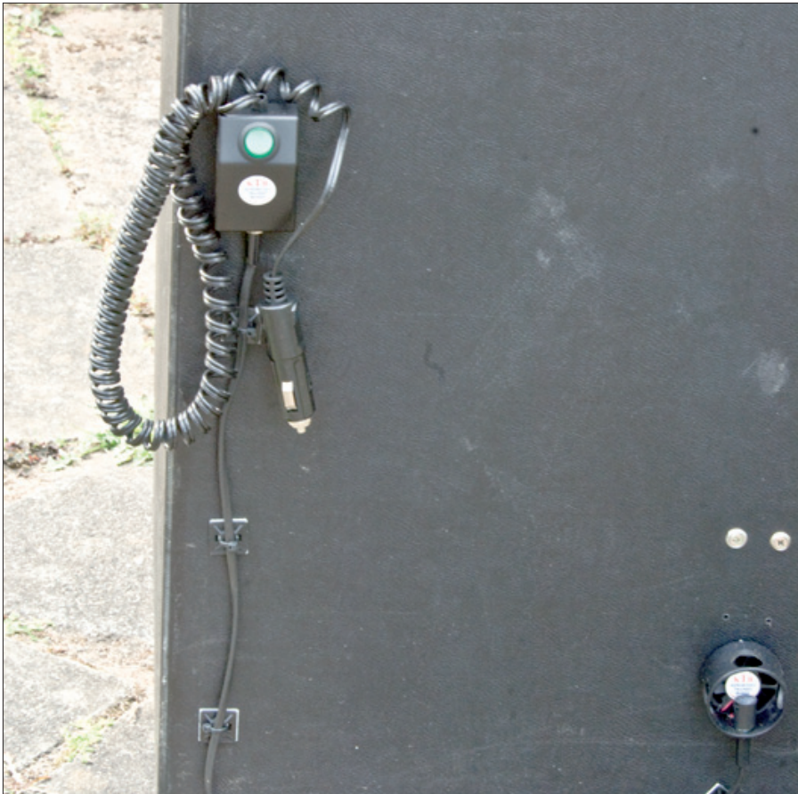
Circular ventilation system in situ
